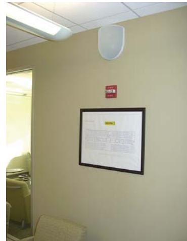
One of the EDICT speakers is located just above the wall-mounted emergency evacuation plan.
